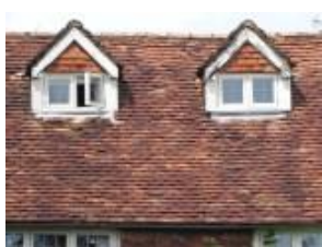
Traditional in Roof
